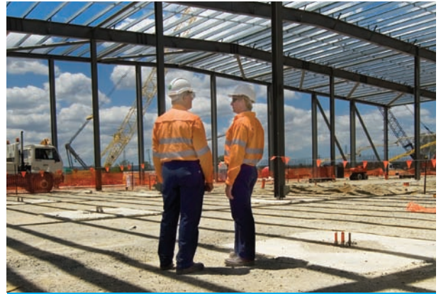
BUNDAMBA ADVANCED WATER TREATMENT PLANT Queensland, Australia
